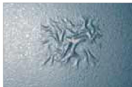
Illustration 2: Corrosion of the machine coating after reaction to a particularly harsh cleaning agent.
